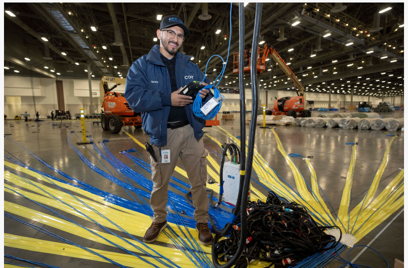
Cox Hospitality Technician Edgar Yanez works on technology installation for vendors in advance of the National Auto Dealers Association Conference held earlier this year at the Las Vegas Convention Center.
