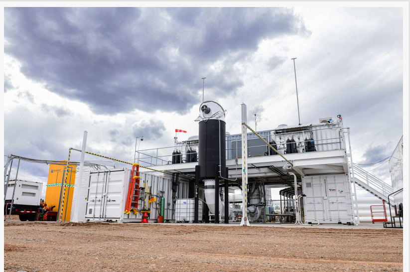
Agile Space's new Animas test stand delivers safe, dynamic altitude based tests of engines over 300 pounds
