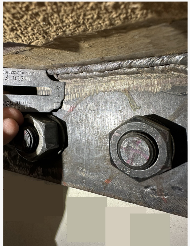
Expert third-party welding inspector from AWSCWI.COM meticulously examining a weld joint for compliance with industry standards.
