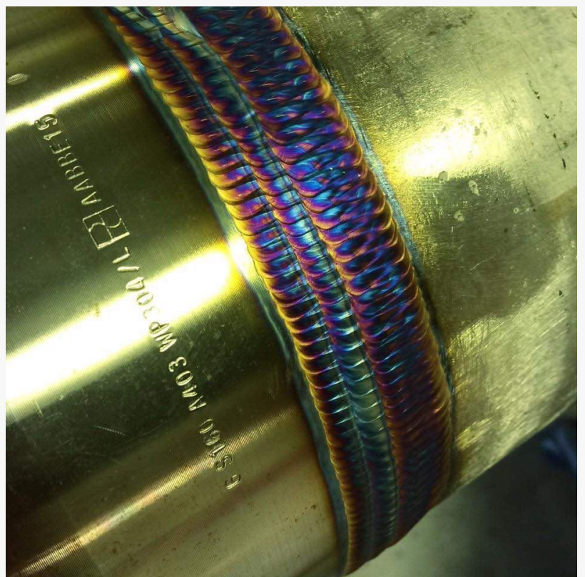
Dedicated AWSCWI.COM welding inspector conducting a detailed third-party examination to ensure weld integrity and compliance.
