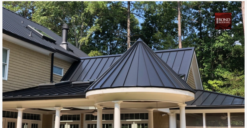
Bond Roofing Metal Roof
