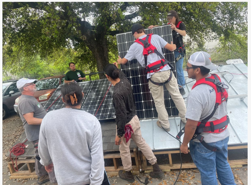
The AYW YouthBuild participants learning how to safely and properly install solar panels and basic circuitry at our campus in Southeast Austin.
