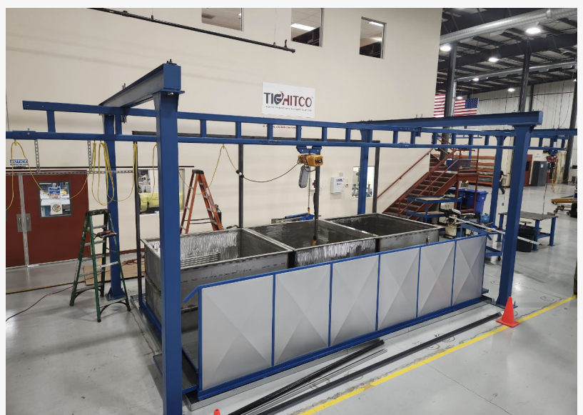
TIGHITCO Alkaline Cleaning Line
