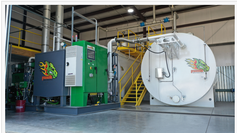
Interior Structure Greasezilla Installation Configuration
