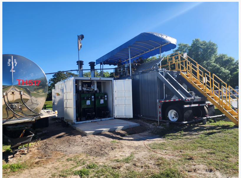
Exterior Greasezilla Installation
