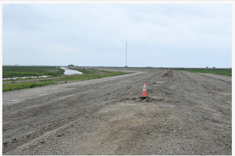
US Army Corps of Engineers, Vicksburg District, awarded Greenup Cajun JV, LLC a construction contract to build hurricane protection structures and to move levees and drainage canals in Louisiana's Plaquemines Parish.
