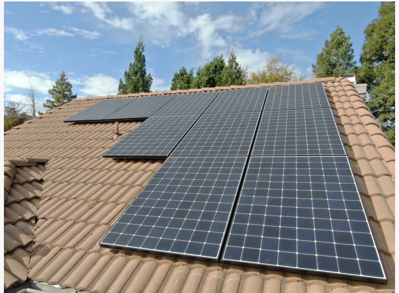
Ambrose Solar Panels
