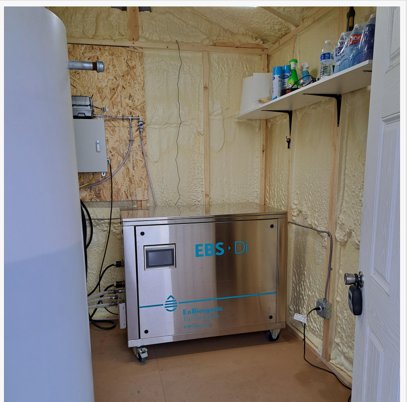
Othello WA EBS-Di Installation
