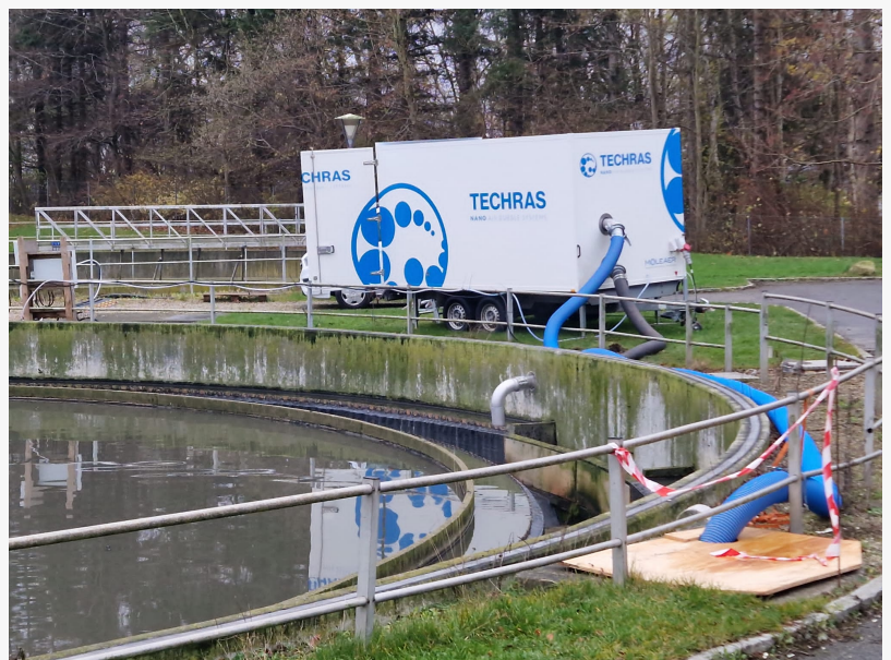
Moleaer Installation at Stavsholt Detail
