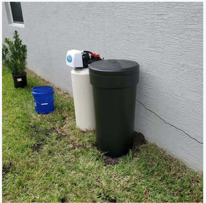
Inside view of local water treatment plant
