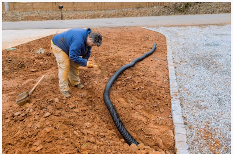
A skilled professional in a blue jacket and khaki attire installs a drainage system to maximize rainwater collection, ensuring adequate water management.
