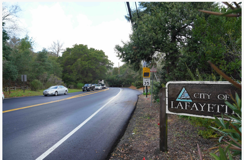
As of today, Lafayette’s Pavement Conditions Index (PCI) is 73. This falls in the Very Good category
