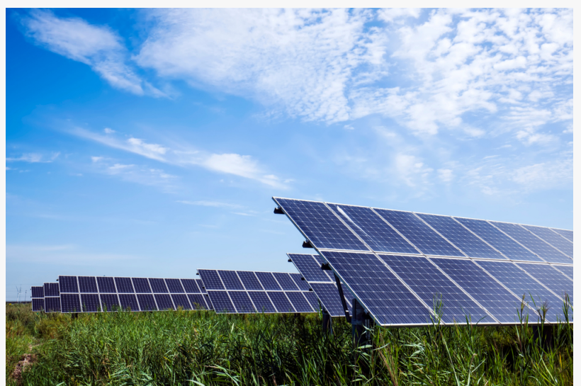
Solar Photovoltaic (PV)
