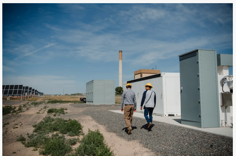
Short-duration battery systems, like the one Platte River has at its Rawhide Energy Station, can harness and dispatch power during off-peak times for two to four hours.
