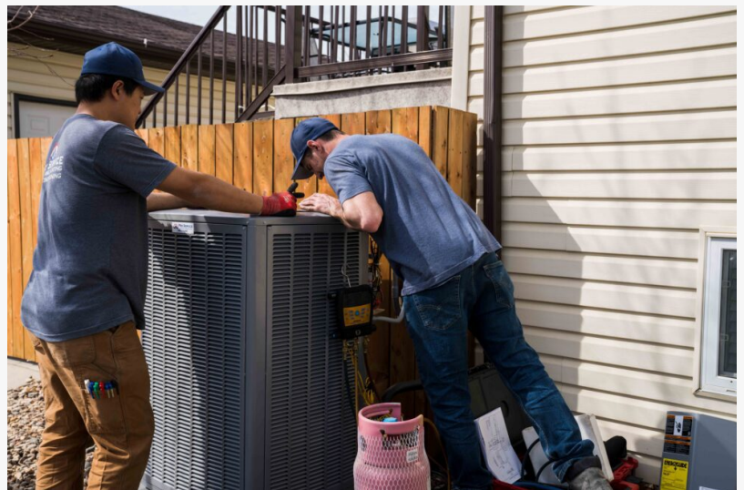
AC Repair Services in Saskatoon
