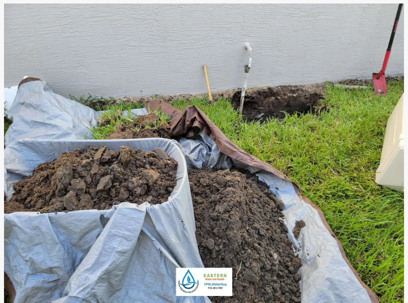
Residential Water Treatment In Port St Lucie - Eastern Water and Health
