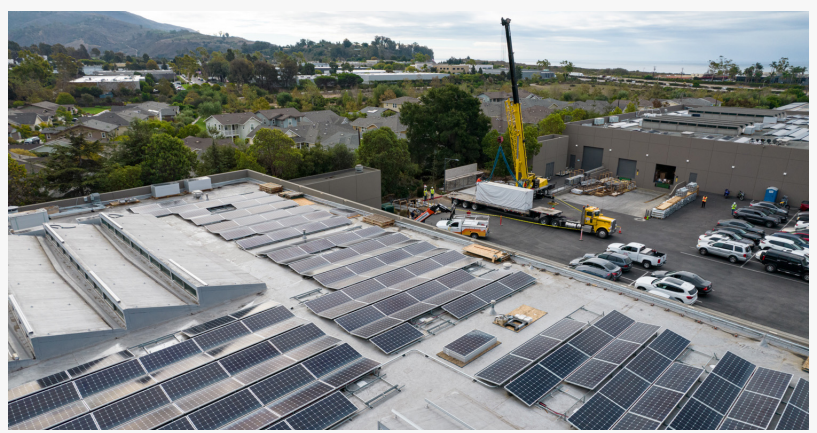
A commercial solar with energy storage system is installed in Carpinteria, California
