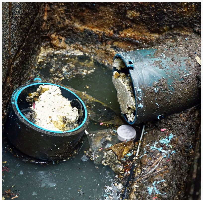
Fats, oil and grease congeal into thick, dense, difficult-to-remove "fatbergs" that eventually clog sewer pipes.
