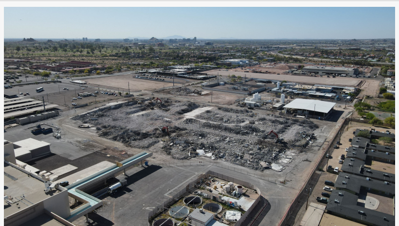
Demolition and recycling of the buildings on the former Motorola campus in Phoenix continues to progress.
