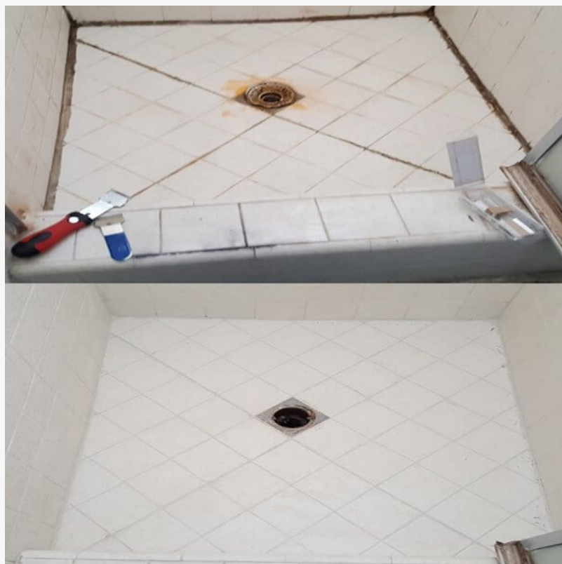
remove and replace damaged and cracked grout from the shower
