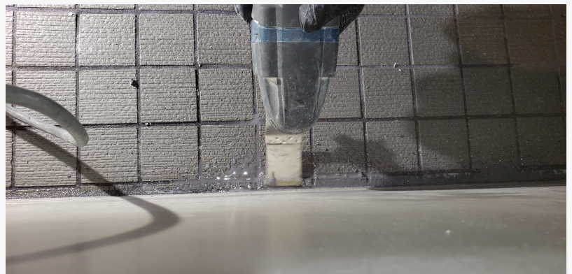
Grout repair, cleaning showed damages and water damage
