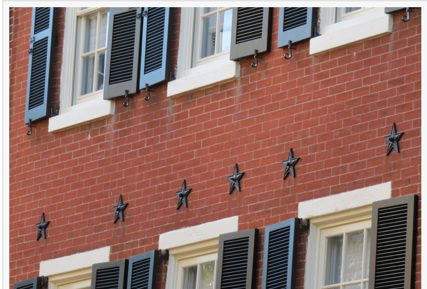
Structural Stars on Historical Brick Building
