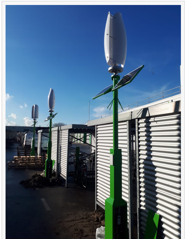
Wind and Solar E-bike Charging Poles
