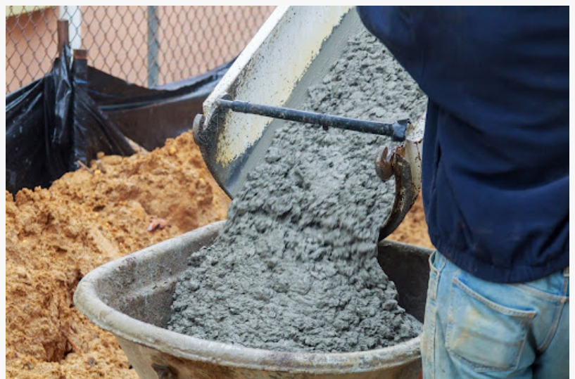
Ready-mix concrete being poured from a truck into a concrete pump at a construction site
