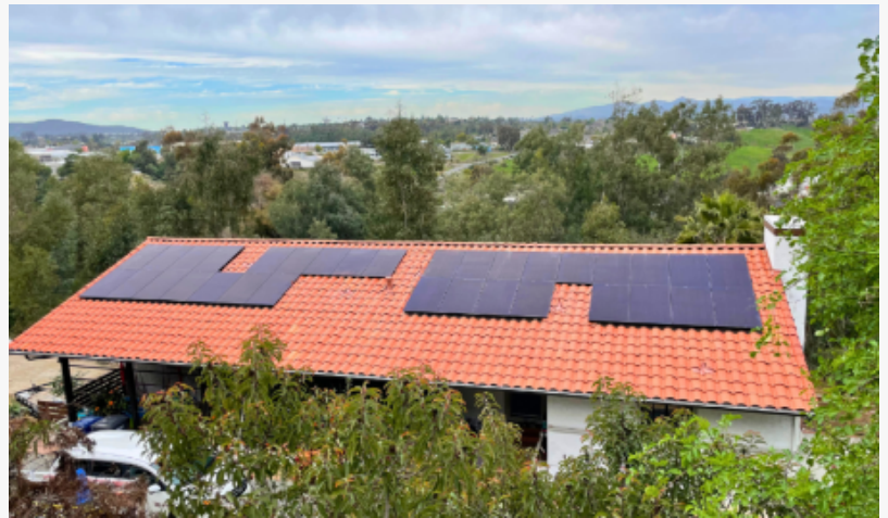
Solar on Tile Roof
