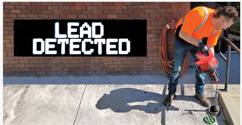
Using Electro Scan's SWORDFISH buried lead pipe can be confirmed from accessing curbstop locations or from inside buildings at the meter.
