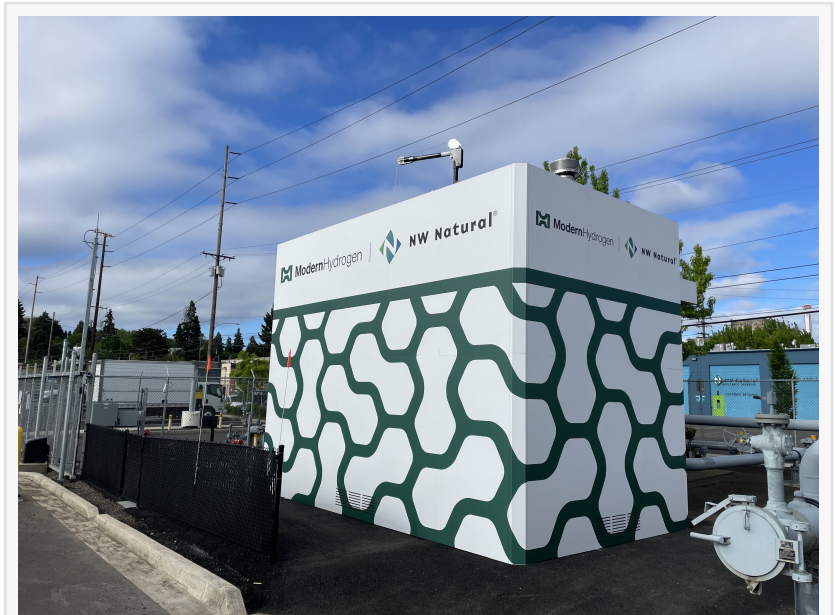
Modern Hydrogen's hydrogen generation unit, located at NW Natural in Portland, Oregon
