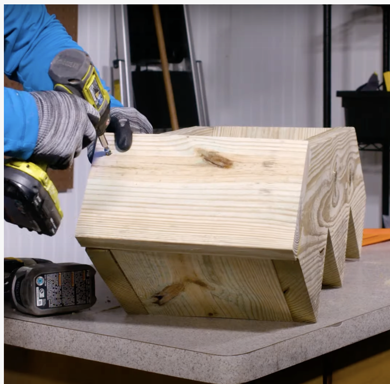
The final step in the construction is to attach the front and back boards to the planter.
