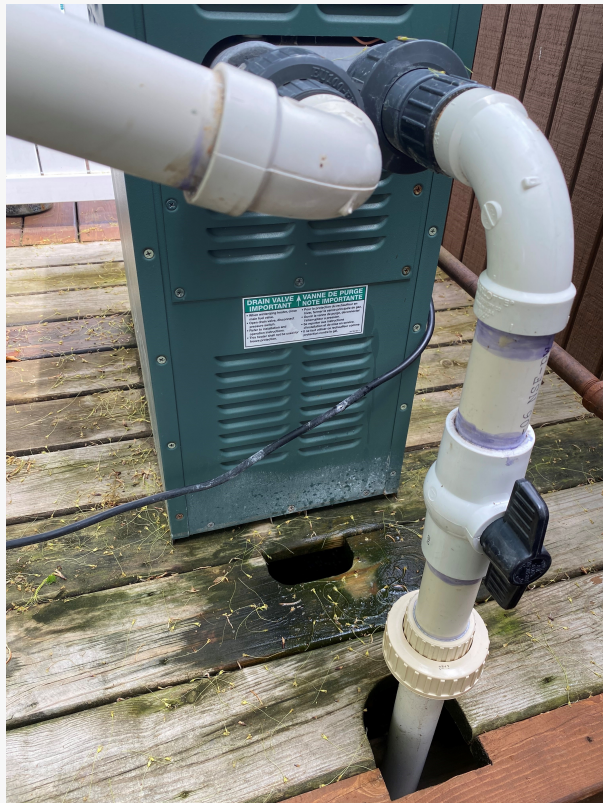
Discolored and rotted wood from leaking pool heater.
