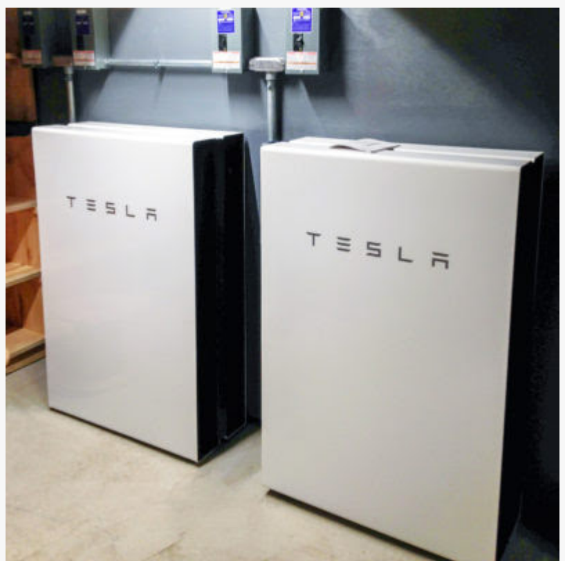
Power wall installed to store the Solar Energy. Reduce the Energy Bill and provide power during a blackout.
