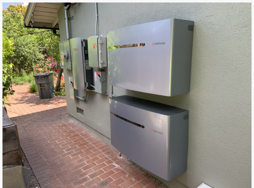
Solar with Battery Backup Solution
