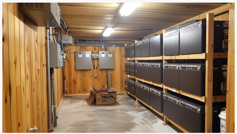
All Things Off Grid - DIY Lithium Battery Pack for Off Grid Energy Storage
