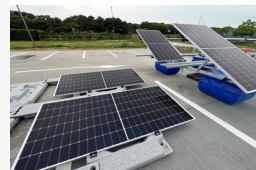
Floating solar panels
