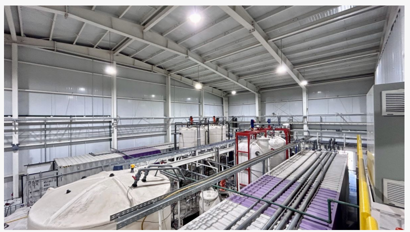
Lithium Extraction Demonstration Plant, Jujuy Province, Argentina, Interior
