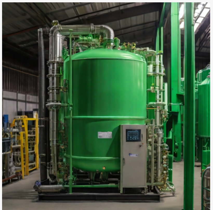
Green Hydrogen Manufacturing Plant
