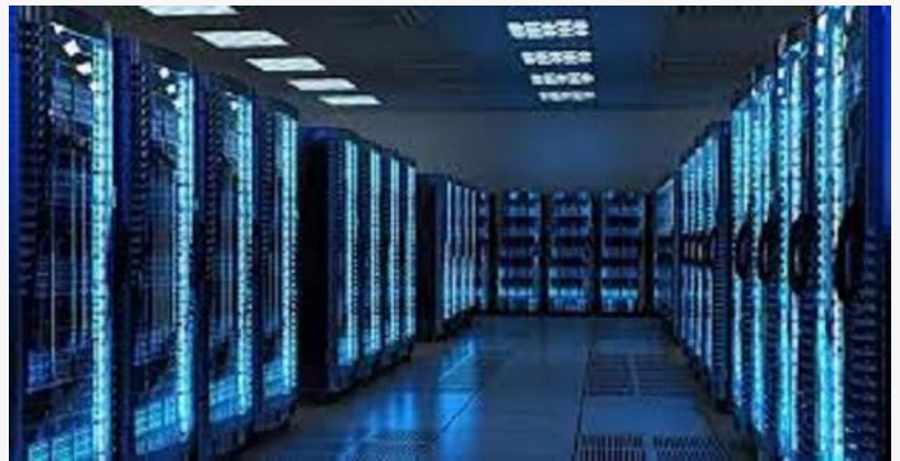
Colocation And Managed Hosting Services Market
