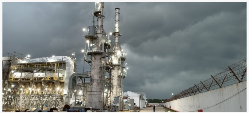
Ducon FGD system in a Chemical Plant in Haldia
