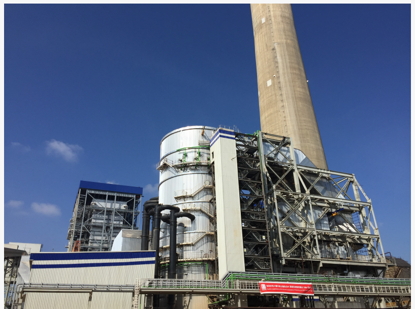
Ducon FGD System in an Industrial Plant
