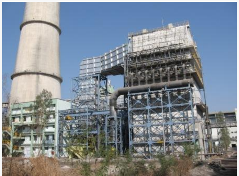
Ducon Seawater FGD System on 500 MW Power Plant
