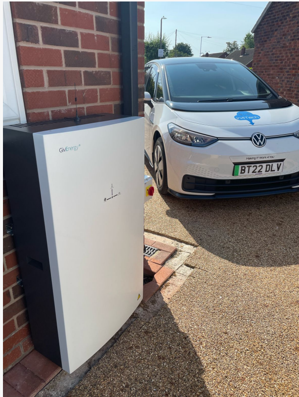
All In One GivEnergy Residential Battery
