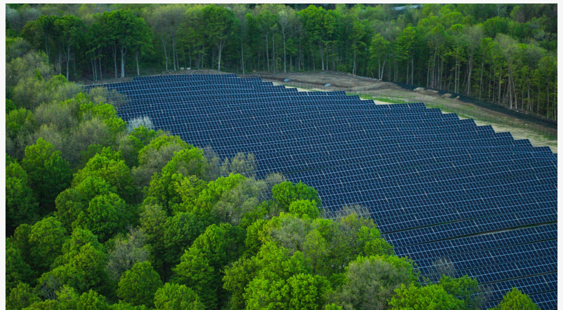
Community solar project by Dimension Energy (Galway, NY)
