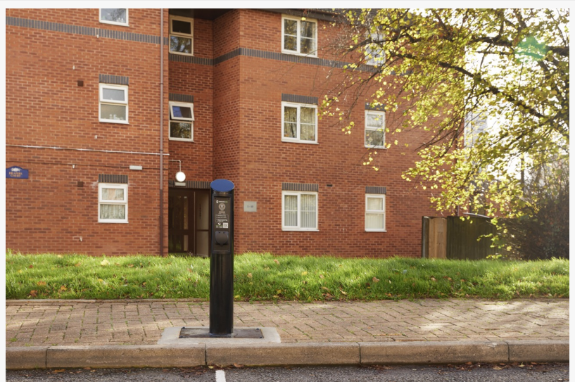
Connected Kerb Chameleon Charging Point
