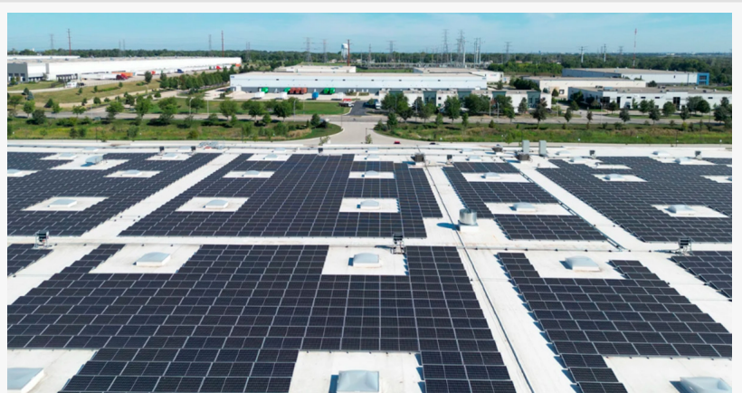
3.09 MW Industrial Rooftop, Romeoville, IL
