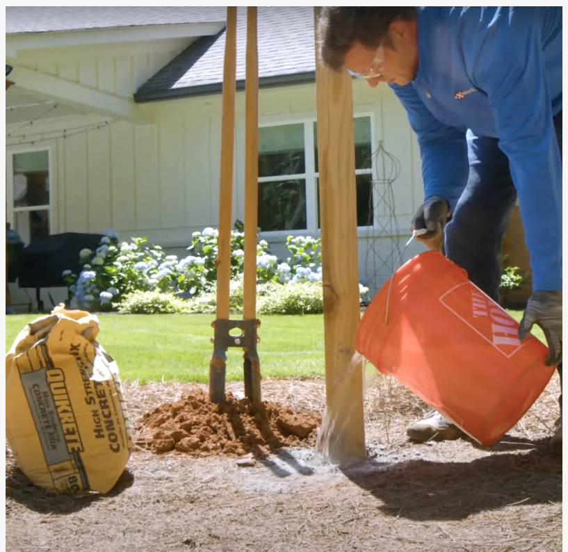
The posts that form the uprights of the living fence are set in concrete.
