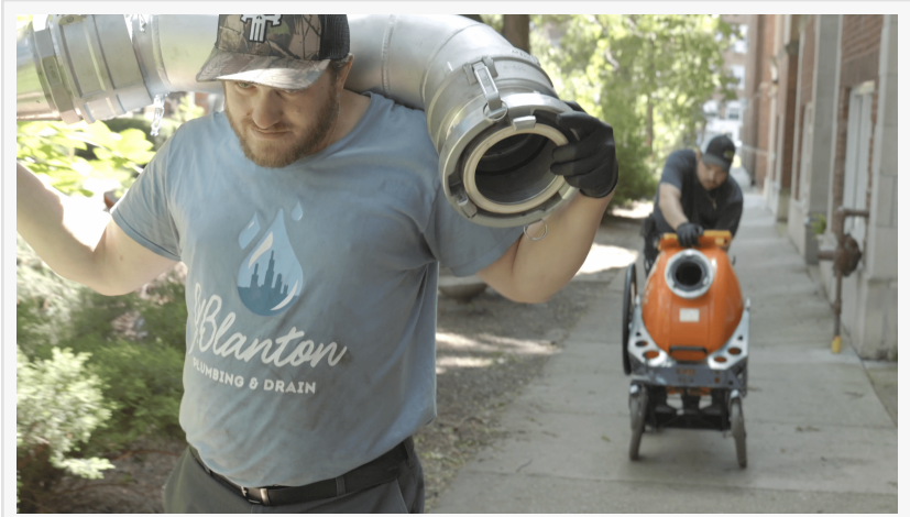
J. Blanton Plumbing team expertly handling a trenchless sewer repair, showcasing their commitment to their sewer repair and sewer line maintenance services.
