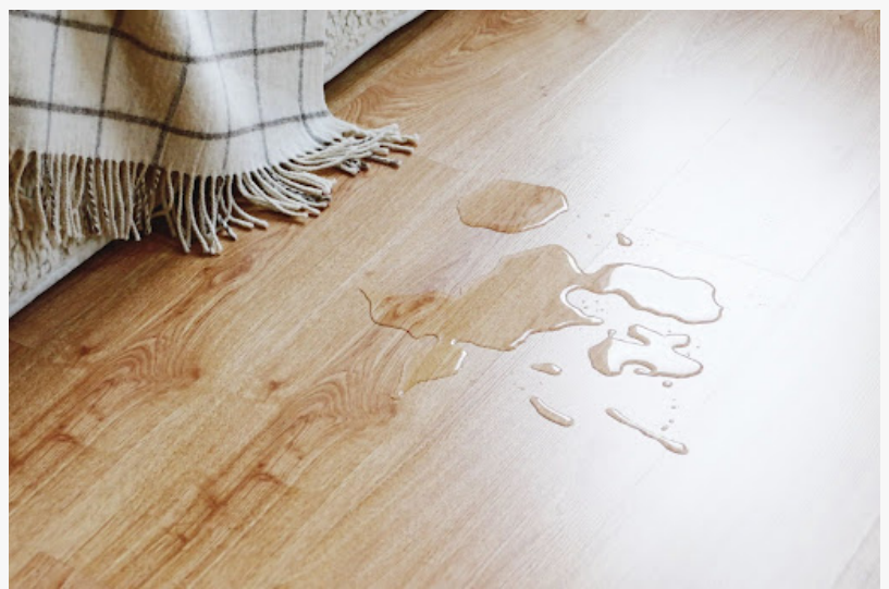
A close-up view of water damage on a laminated floor in a living room, with visible water pooling and warping of the laminate boards.
