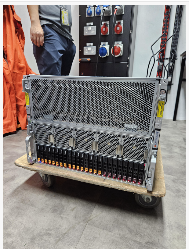
a Supermicro GPU Server System, powered by Nvidia H100 GPUs, installed on site by team Bossjob in Singapore as part of its trial to build a proprietary recommendation ML model on a private cloud.
