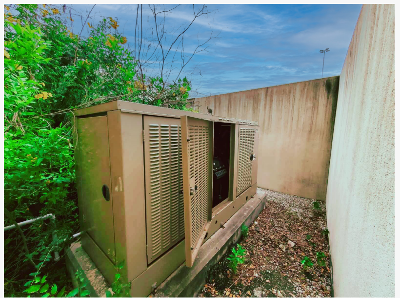
CS Mechanical Now Offers Residential Generator Installation and Maintenance
