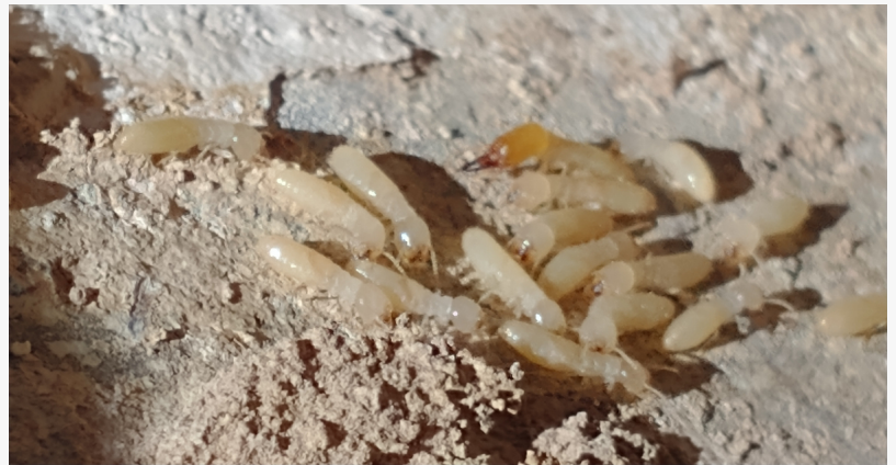
Termites on Stucco as Taken by Chris Fitzgerald, Owner of Critter Getter Pest Control
