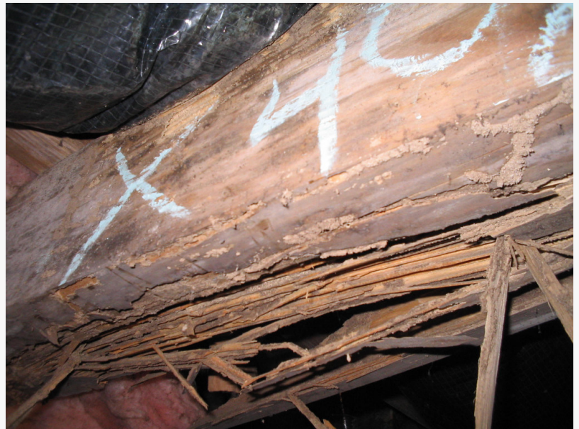
Termite Damage in Virginia Beach
