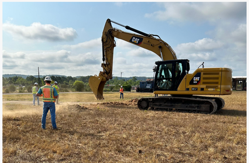
Workers started excavation at the Hermes site in Oak Ridge on July 17, 2024
